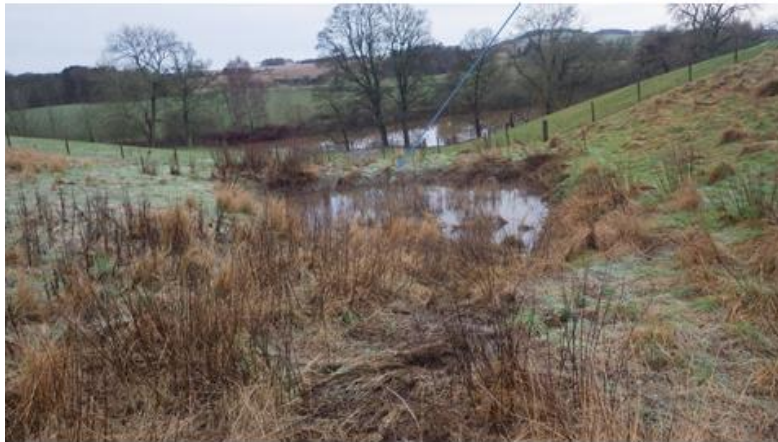
Bund with high flow drain and settlement pond
