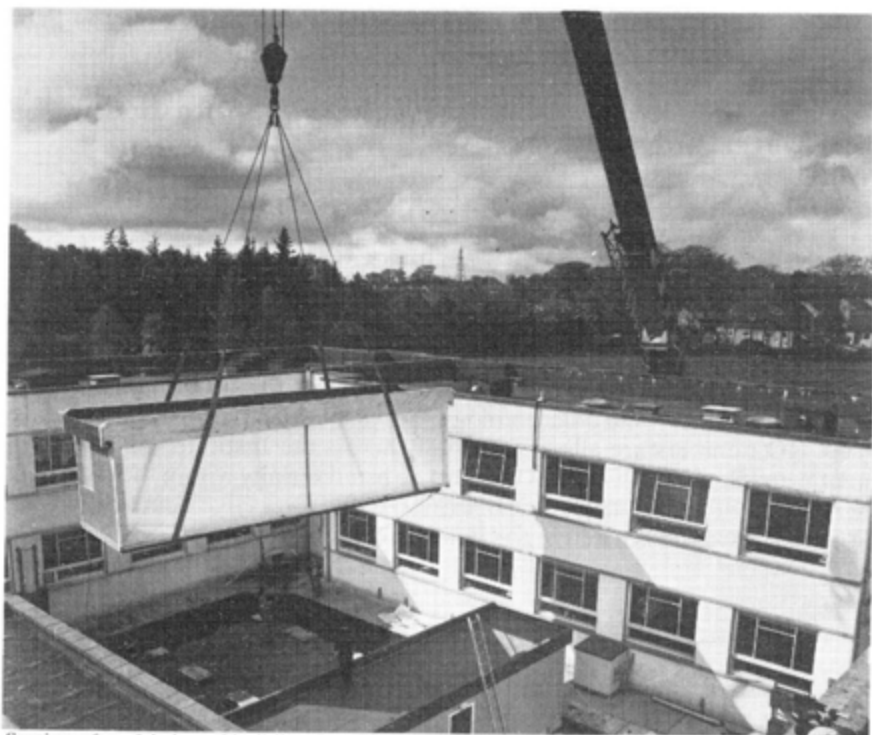
Section of prefabricated building for offices for the Department of Peat and Forest Soils being lowered by crane into the central quadrangle of the main building.
